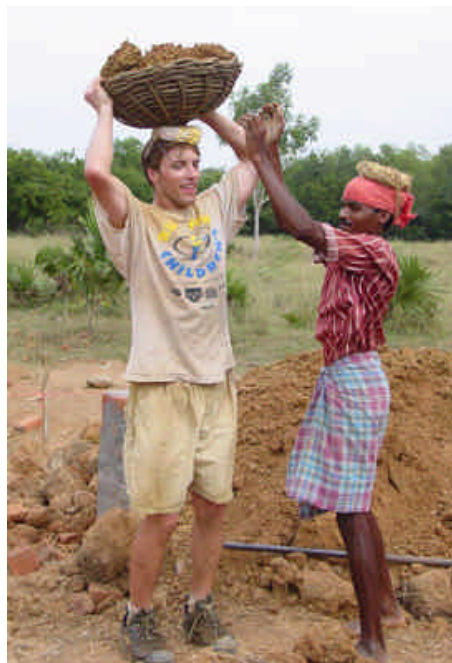
Willy from the University of WA helps carry dirt away from the pit that will hold the USA Pavilion's underground cistern.
